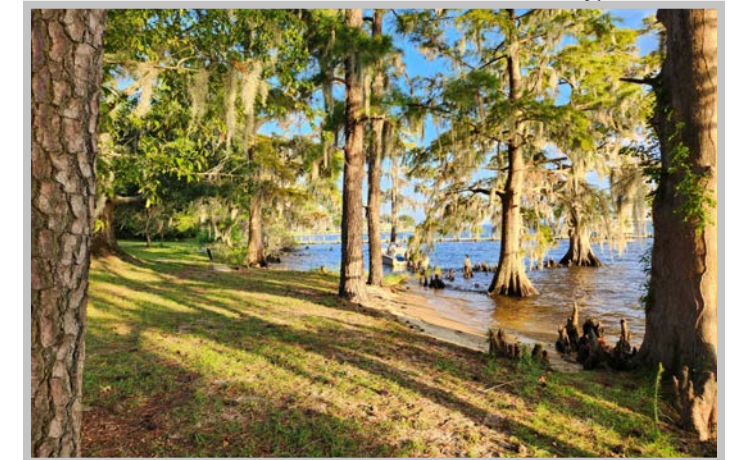
Minor Shoreline erosion. Shoreline receding closer to pine tree. Source: Team picture on 09/12/2023
