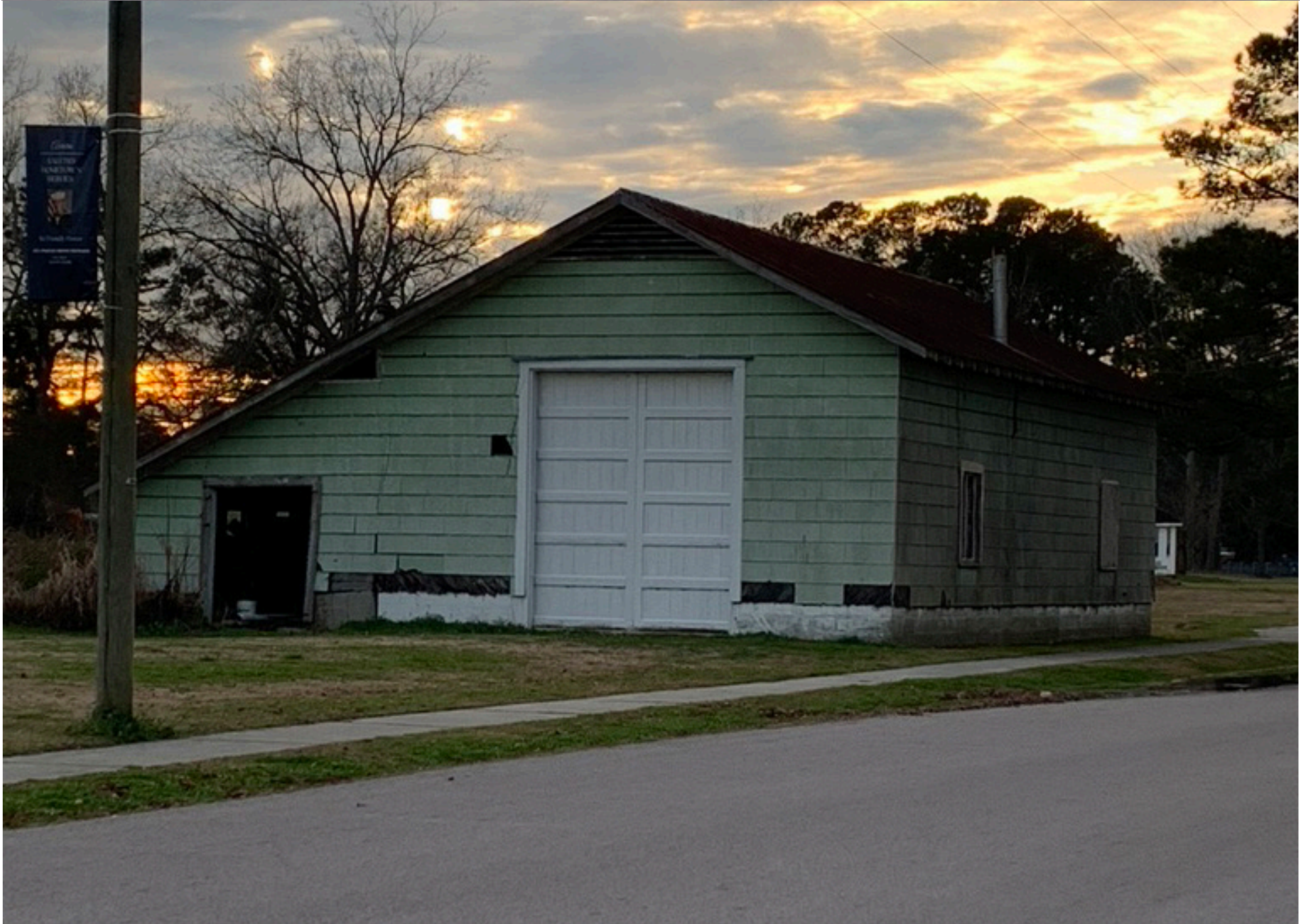
Representative examples of substandard structures near the waterfront that the Town of Aurora would like demolished
