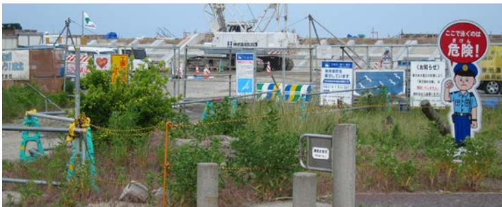
Increasing the height of sea wall in Sendai, Japan after the 2011 earthquake and tsunami
